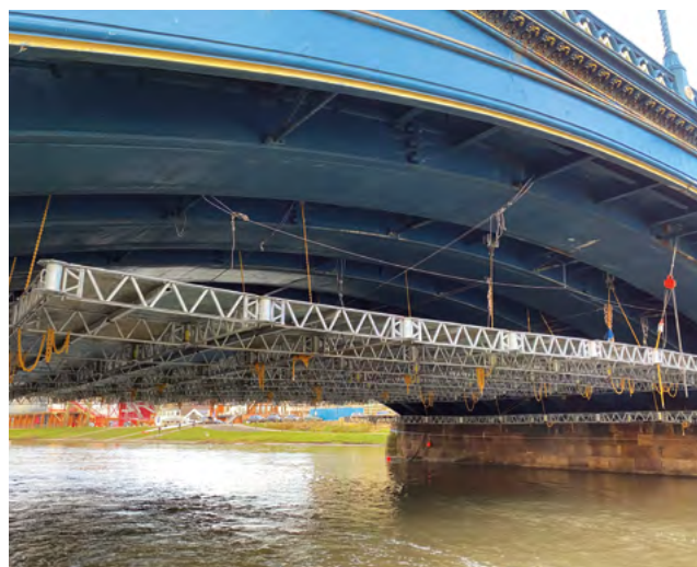
► Trent River Bridge (UK): QuikDeck provides high working safety thanks to high load capacity of the suspension chains
